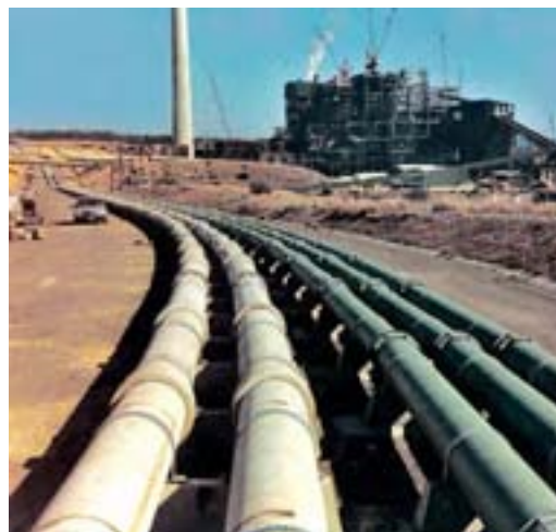
Pipes in Australia; the pipes are connected by "Victaulic" couplings
