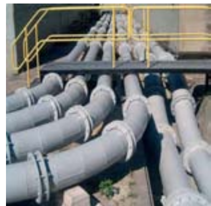
Pipe for several units running to the central disposal site in Brasil
