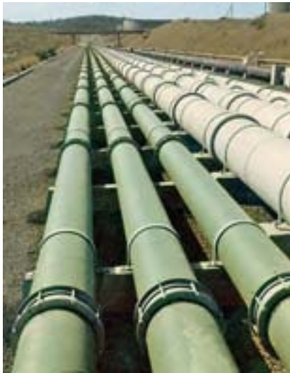
Wear protection for hydraulic and pneumatic pipes
