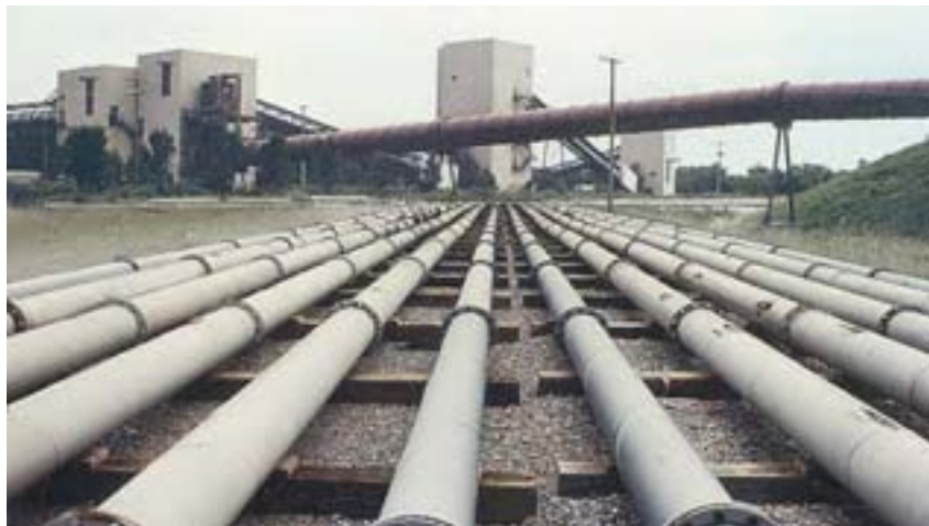
Reliable protection of pipe. ABRESIST fused cast basalt as time-tested solution for the transport of wet ash in the USA (250 mm diameter).
