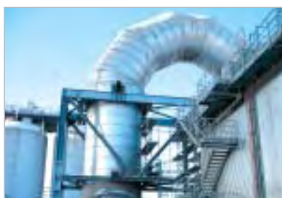
Clinker dust transport pipe in a German cement plant
