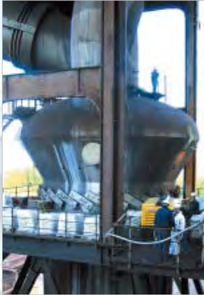
The KALCRET spraying technology allows quick and reliable lining of large surfaces; this illustration shows lining of a scrubber in a steel making plant with KALCRET-S hard compound
