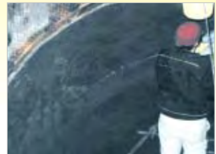
Raw meal duct in a cement plant
