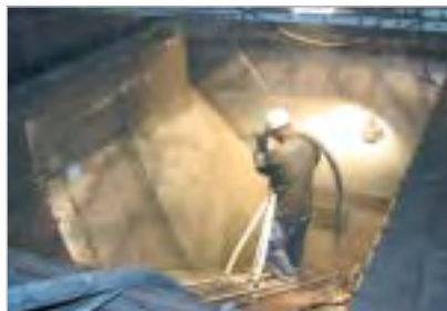
Lining of a wind box underneath a sintering belt in steel works
