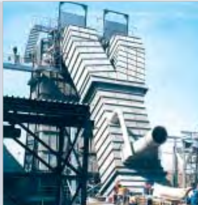
Lining of a cooler pipe that handles clinker in a cement plant with KALCRET-BNY hard compound; the prefabricated shaped elements with integrated insulation have been provided with mechanical fastening system
